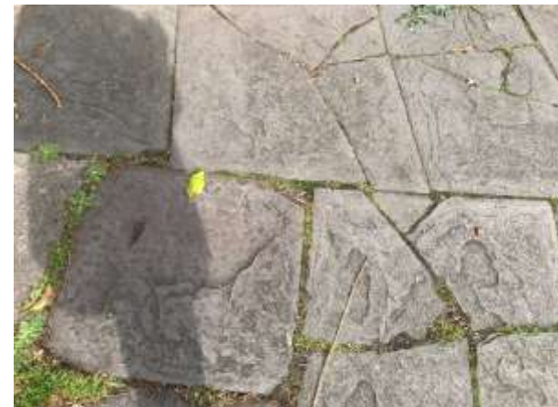
Uneven paving corner of City Road and Ashley Road
