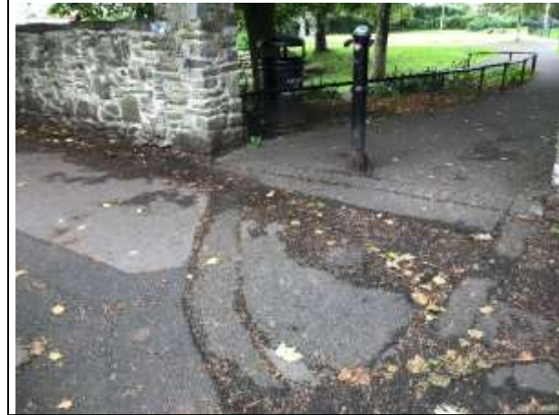
Uneven tarmac path at the entrance to St Paul's Park
