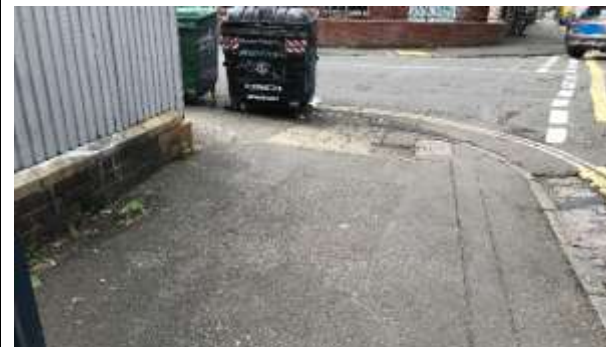
Corner of Ashley Road and Brigstocke Road, uneven sunken pavement on the corner.
